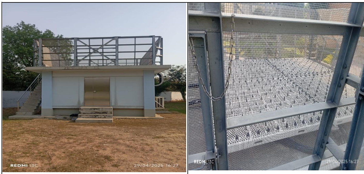
Fig.3.2.2. Wind Profiler installed in Islamabad
