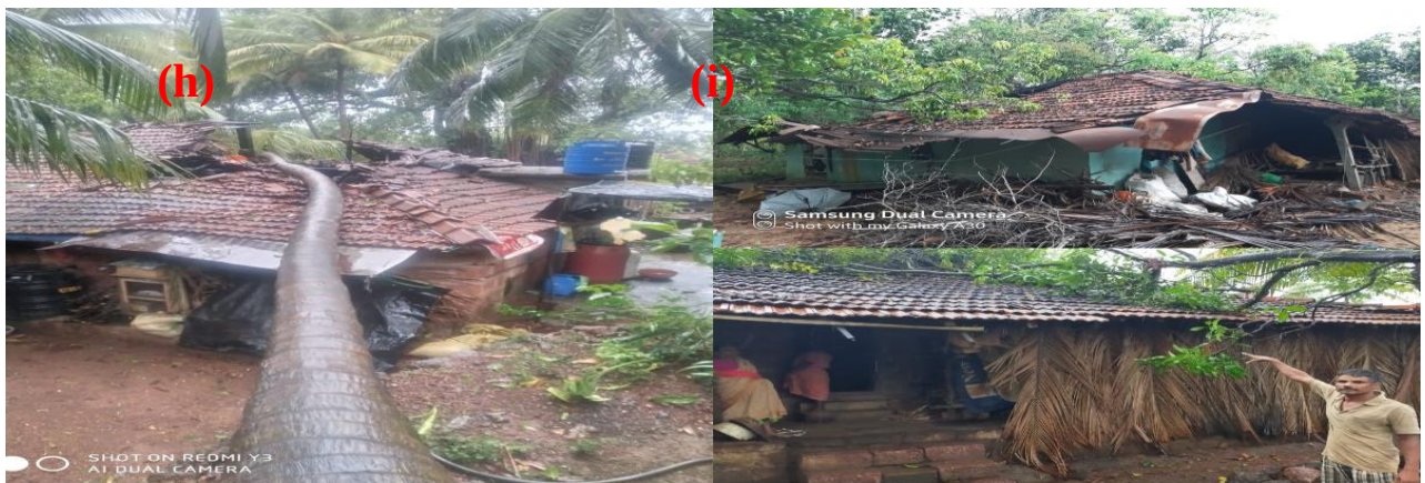
Fig. 2.4.10 (h-i) Houses damaged from Sindhudurg Dist. Maharashtra (Source: NDRF)
